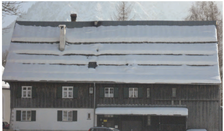
Pict. 4: A sheet system divides up the large forces appearing into several smaller ones. Therefore, only small snow masses start to move.
