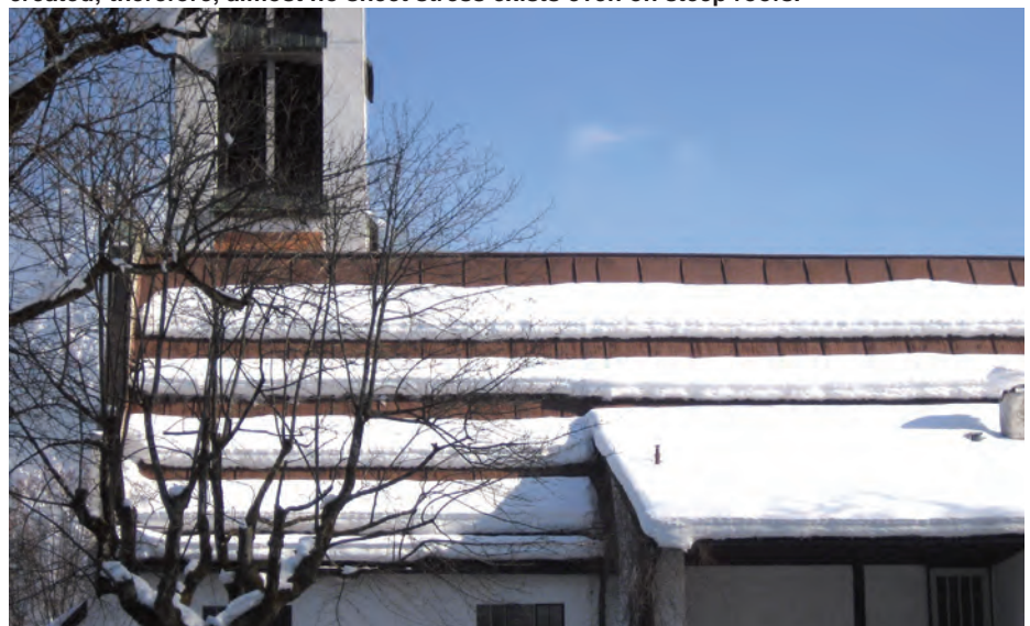
Pict. 4: Due to the sheet distribution of tubes, individual snow fields are created; therefore, almost no sheet stress exists even on steep roofs.
